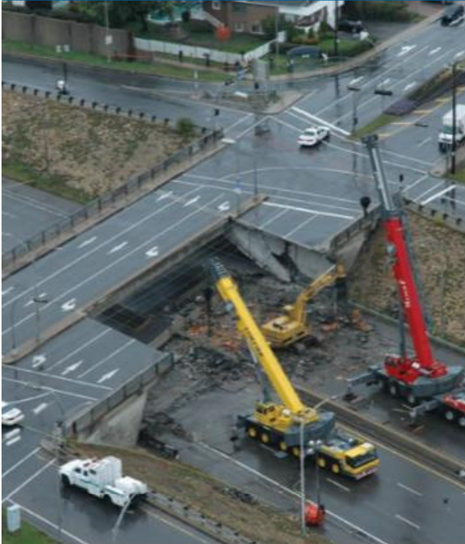
Collapse of the (concrete) De la Concorde Overpass, Montreal, 2006
