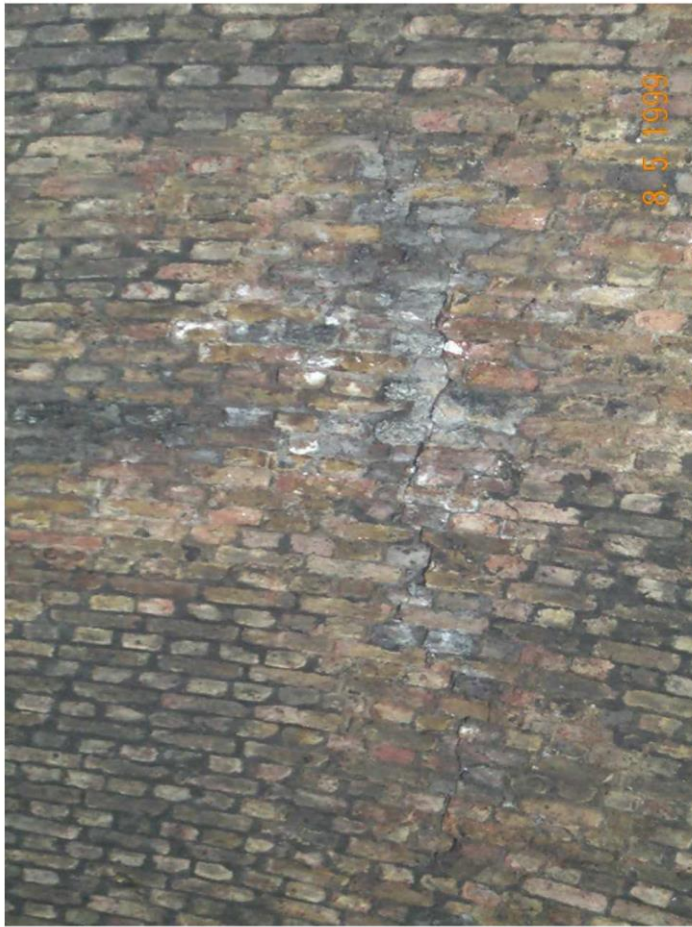
Photograph 2C.31: Longitudinal crack in barrel arch maximum width >5 to 10mm (Severity rating K)
