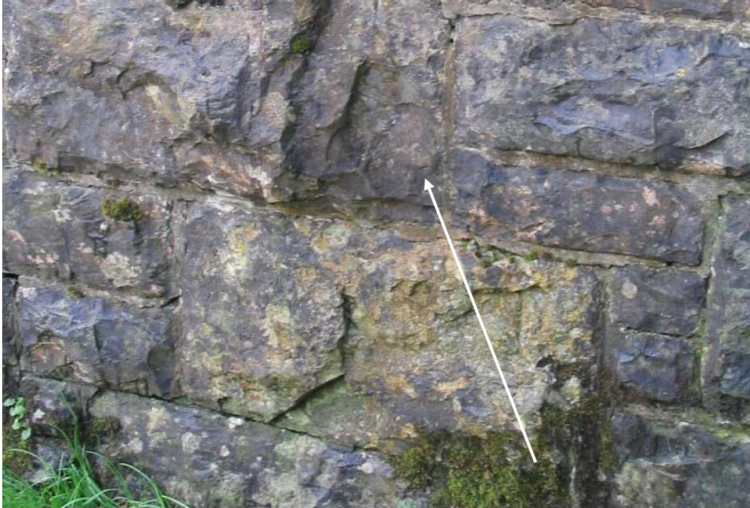
Photograph 2C.24: Example of a stone wing wall where the depth of the defect \geq 20\text{mm} (Severity rating D)
