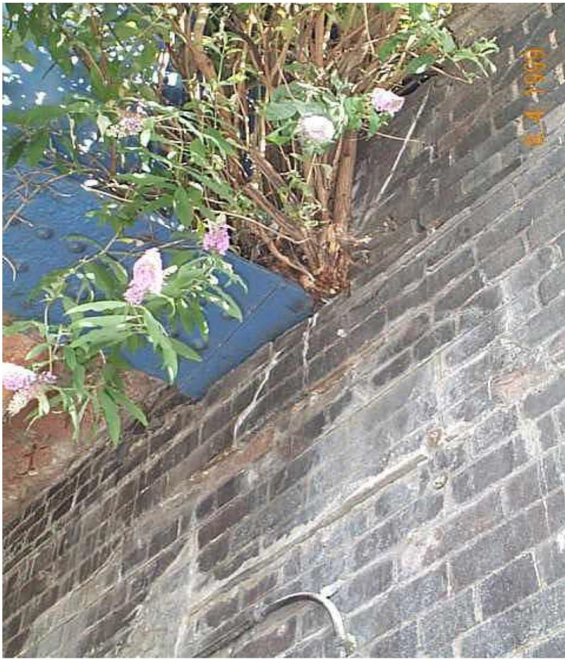
Photograph 2C.17: Bulging with associated cracking to be scored twice, once as severity rating F (bulging) under general masonry and once as severity rating N (horizontal crack, maximum width/displacement 5mm to 10mm) under cracked masonry
