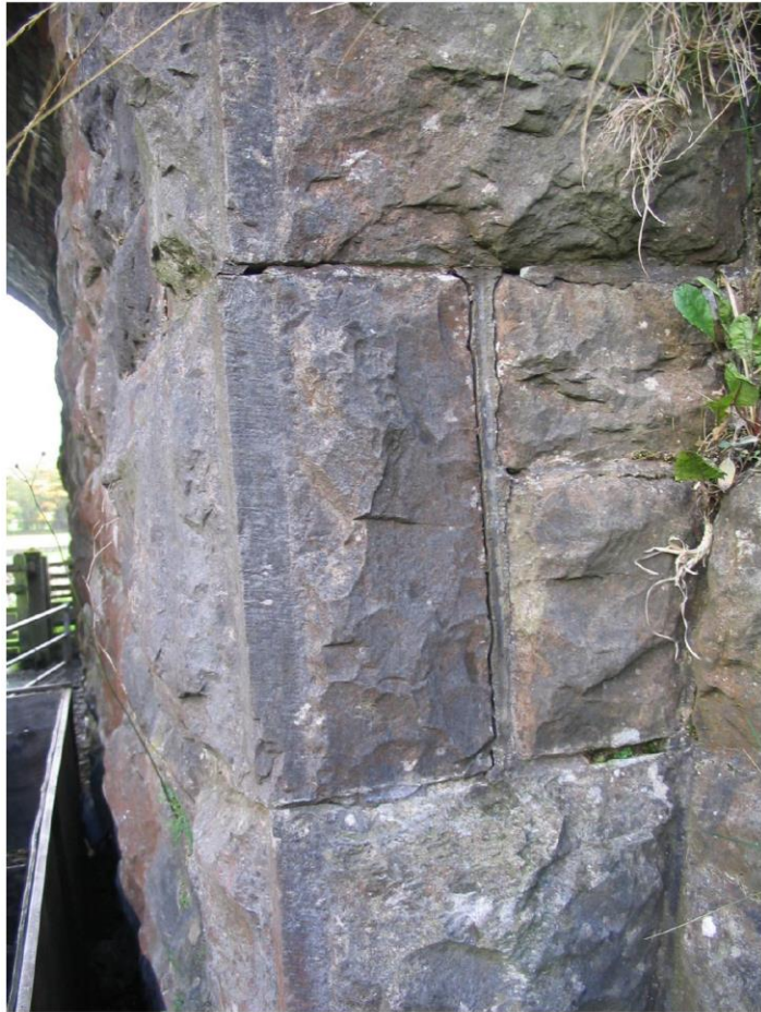
Photograph 2C.29: Example of a stone abutment with a displaced block (Severity rating Ex)
