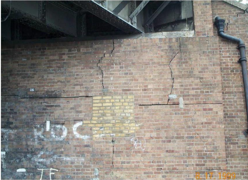
Photograph 2C.33: Abutment with horizontal and vertical cracks wider than 10mm (Severity rating O and L respectively)
