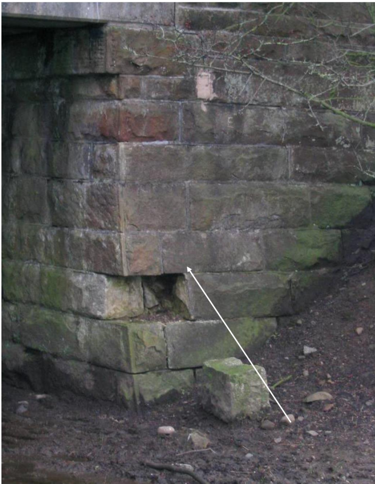
Photograph 2C.27: Example of an abutment with missing stone (Severity rating Ex)
