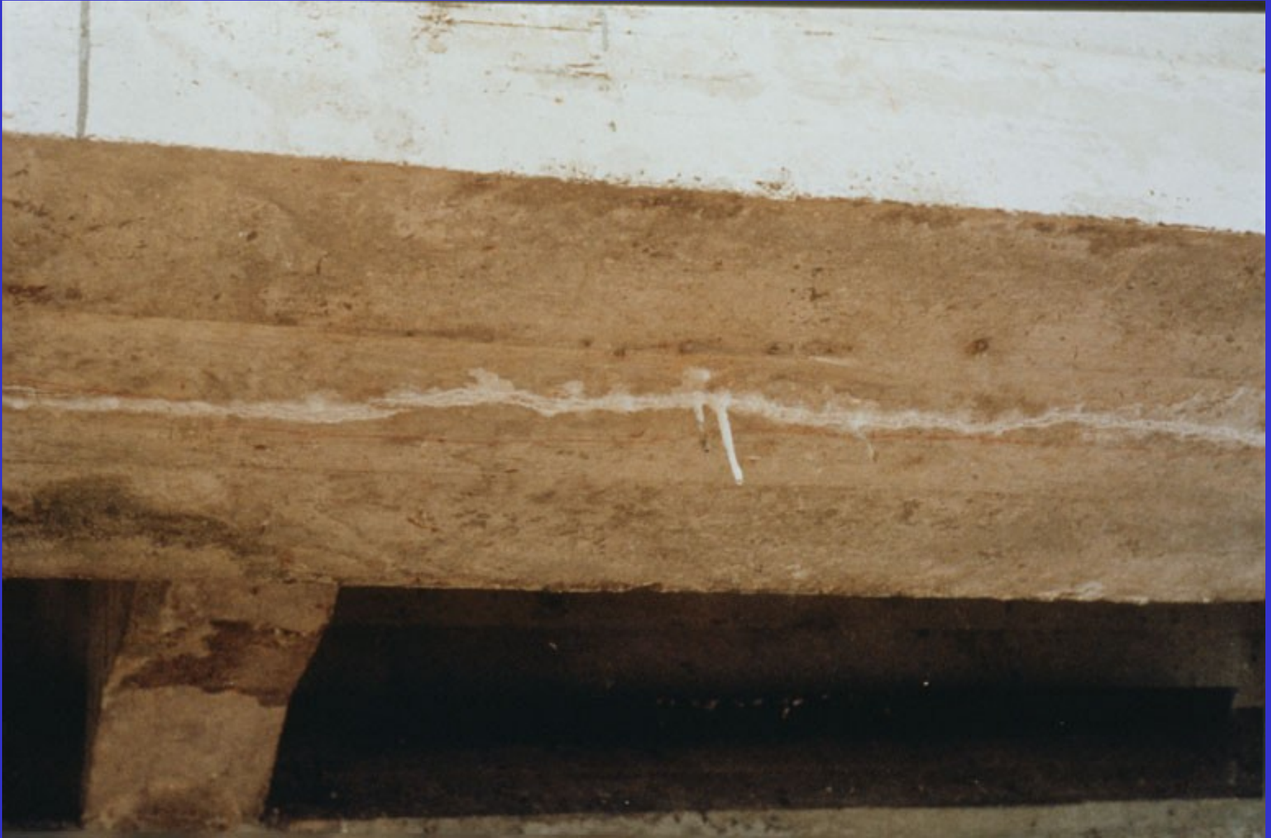
Crack with stalactite at the soffit of the toe of a beam
