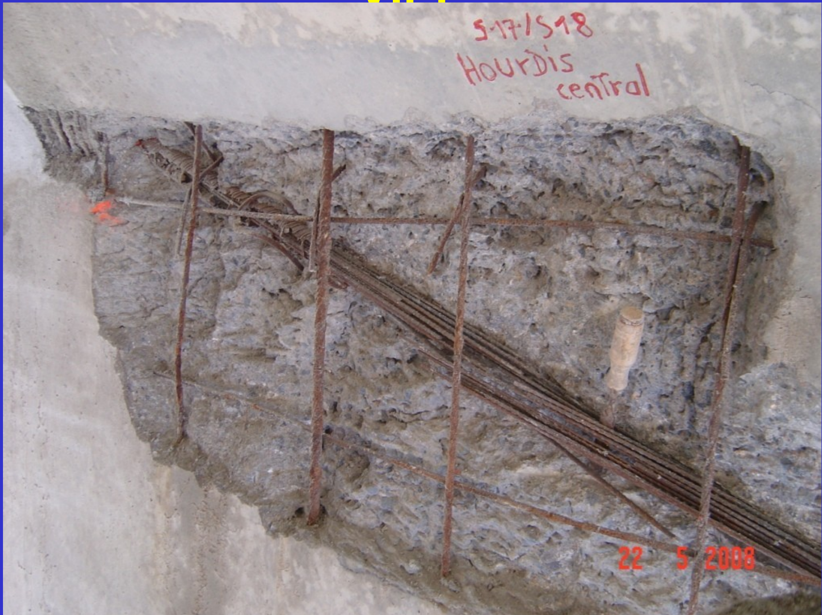
Example of broken wires due to SCC (KA system)
