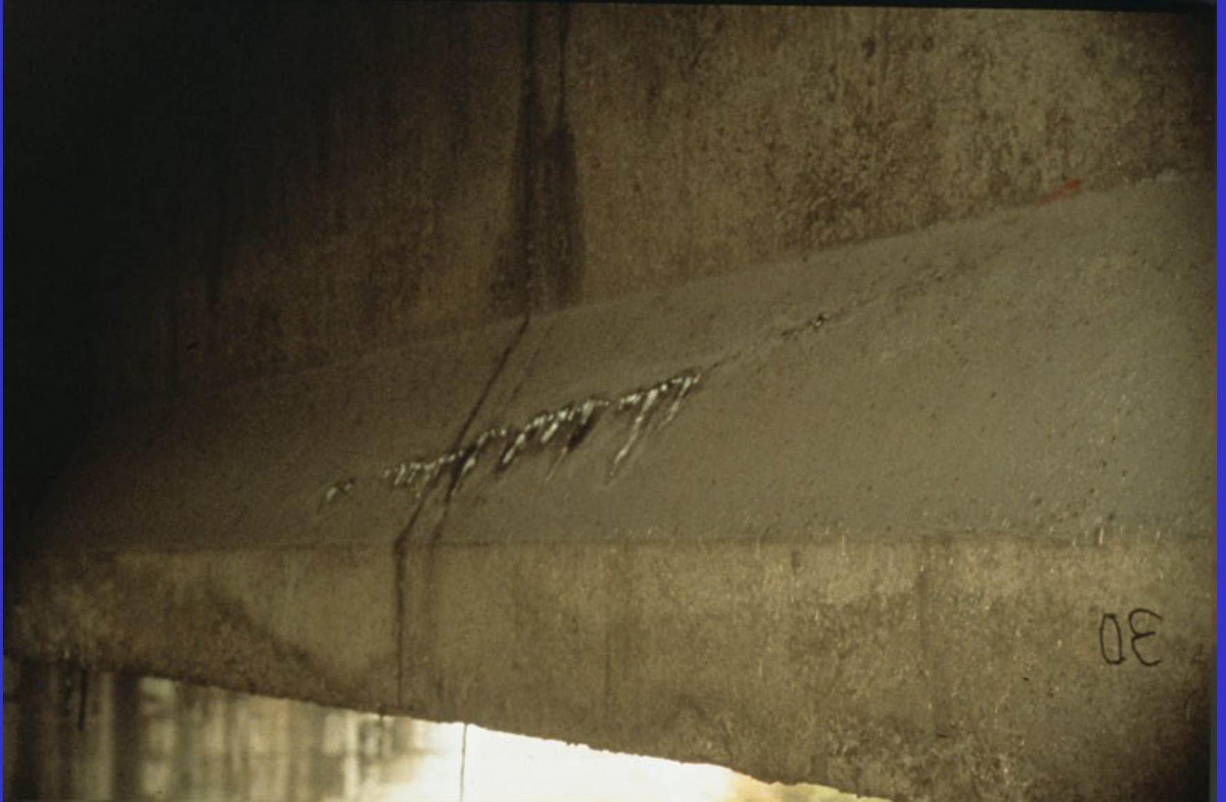
Active humidity in a crack on the toe of a beam...
