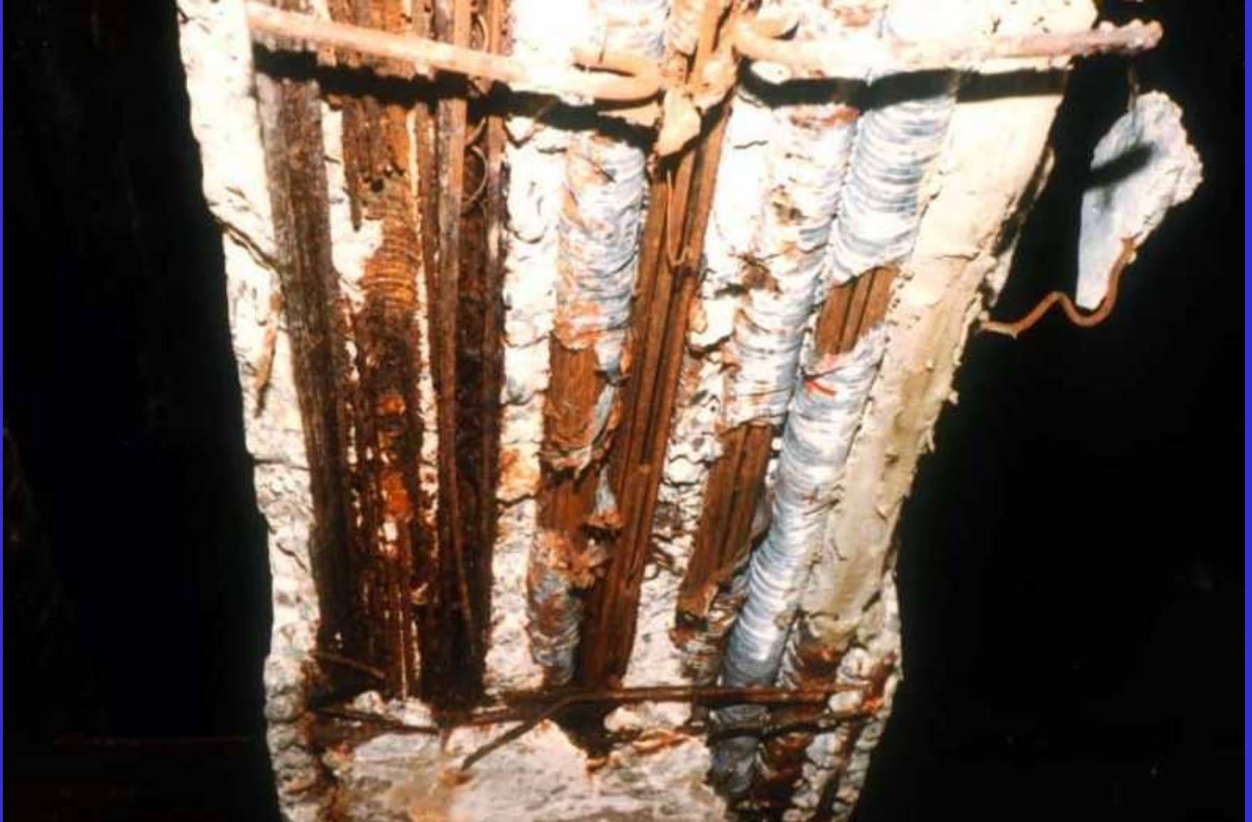
General corrosion of tendons
